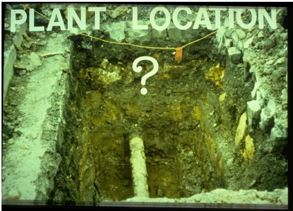
Figure 1. Example of pipe buried in wet clay
