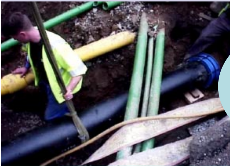
A typical tangle of pipes and cables under our city streets that can result in expensive third party damage
